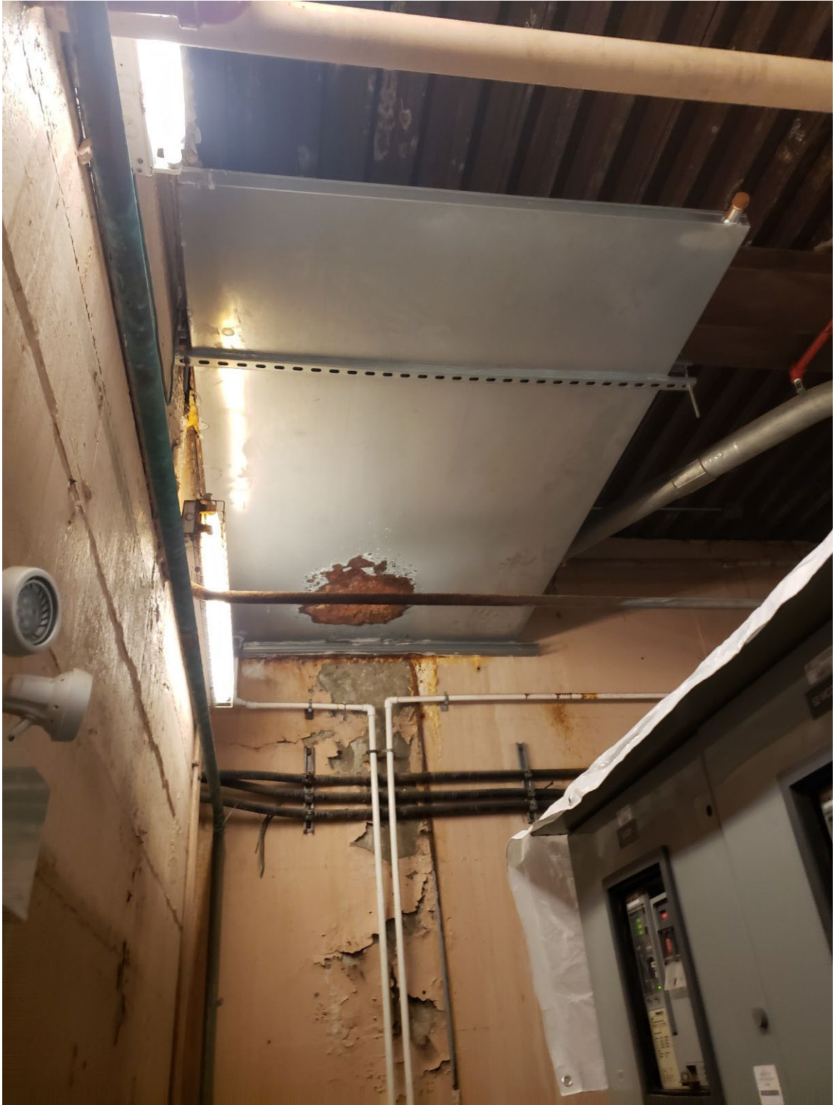
Figure 8: Water Infiltration within the Electrical Vault; Failure in Roof Construction
