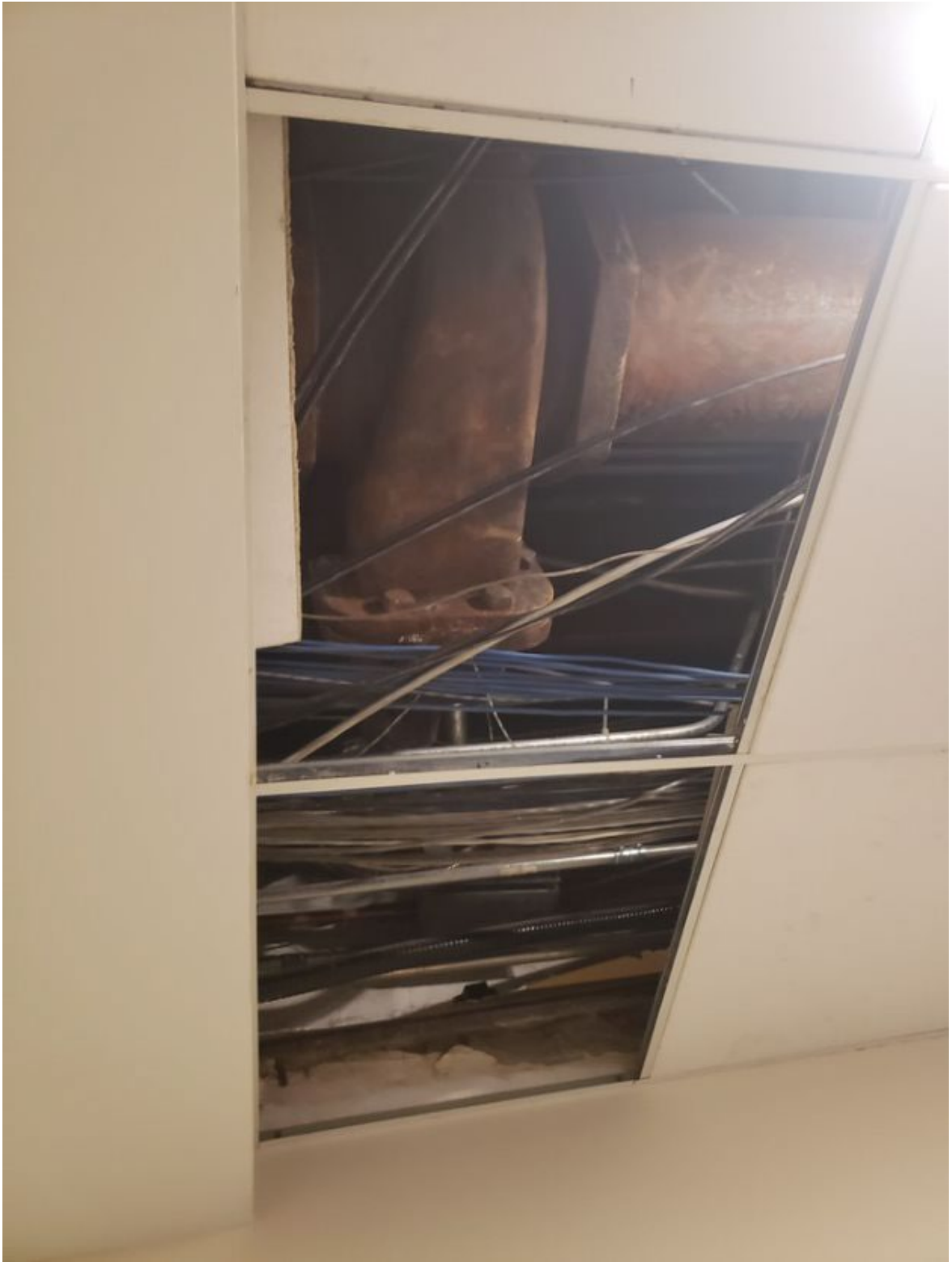
Figure 12: Original Eight-Inch Diameter Main Steam Isolation Valve, Limited Access for Repairs and Would Result in Major Disruption of Services
