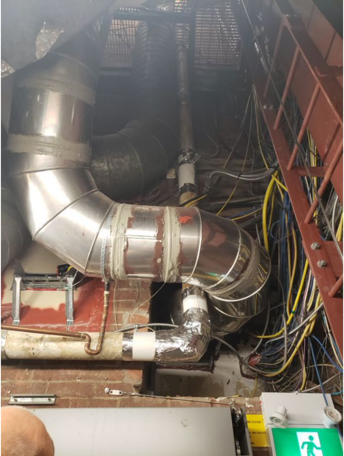
Figure 6: Masonry Shaft, Existing Fire Damper was Compromised by Decades of Cabling
