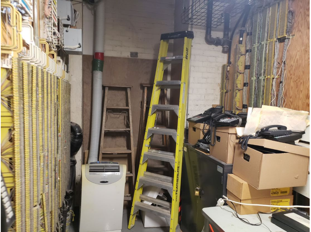
Figure 9: Abandoned Telephone Panels and Primary Distribution Cables are Inaccessible for Removals
