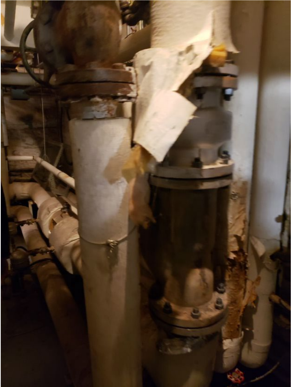
Figure 11: Main Steam Distribution Piping
