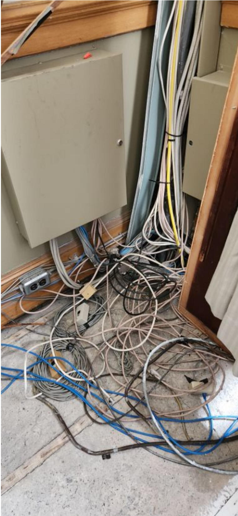
Figure 4: Congested Vertical Raceways - Typical
