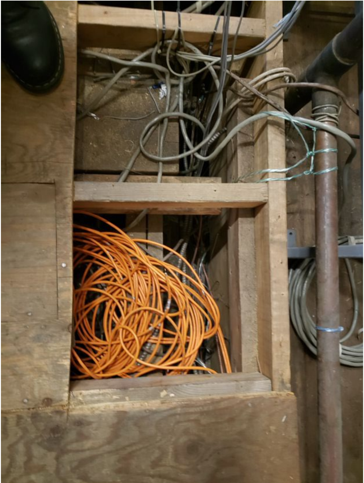
Figure 13: Concealed Cables Running in Vertical Vent Shafts between Floors without Fire Stopping - Typical
