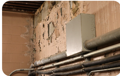
Pipes located in the basement. Leaks and flooding are prevalent with the current pipes.
