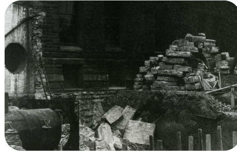
Construction of the north wing in 1910. Portions of the back wall had to be removed to incorporate the new addition.
