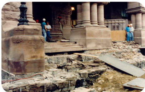
Extensive restoration of the exterior stonework and main entrance in the 1990s. As sandstone is a soft stone, it erodes very quickly.
