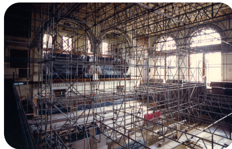
Floor-to-ceiling scaffolding in the Legislative Chamber during renovations in the 1990s. A complete restoration of the space was completed.
