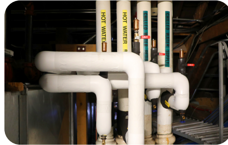
Steam pipes in the attic. Steam heat is inefficient and problematic in the summer months.
