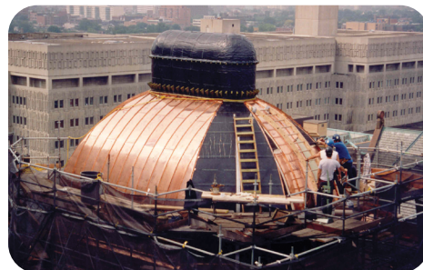
Copper roof being installed in the 1990s. Over 51 tonnes of copper were used on the building's exterior.
