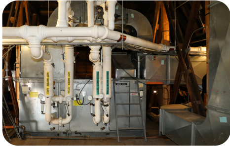
Current HVAC units in the attic. They are close to the end of their lifecycle and need to be replaced.
