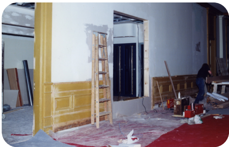
Installation of the Broadcast and Recording booth on the 3 rd floor in the 1980s. Cameras and lights were also installed in the Chamber.
